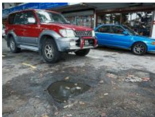
Potholes along Jalan Aminuddin Baki, TTDI getting worse
